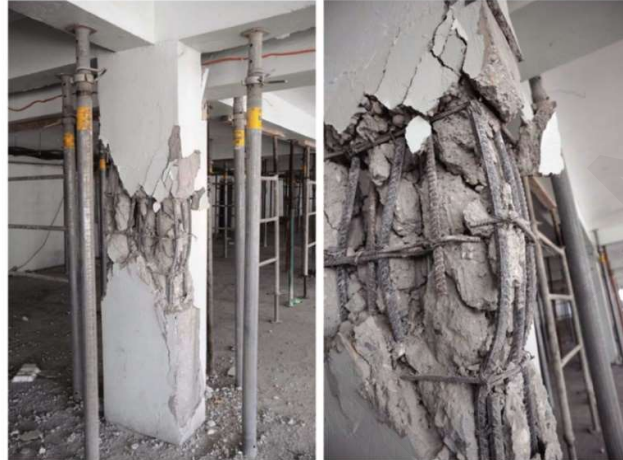
Figure 1.3 : Shear failure of columns in the parking garage of the Digicel building (note the 90-degrees hooks in right photo, Paultre et al., 2013).
