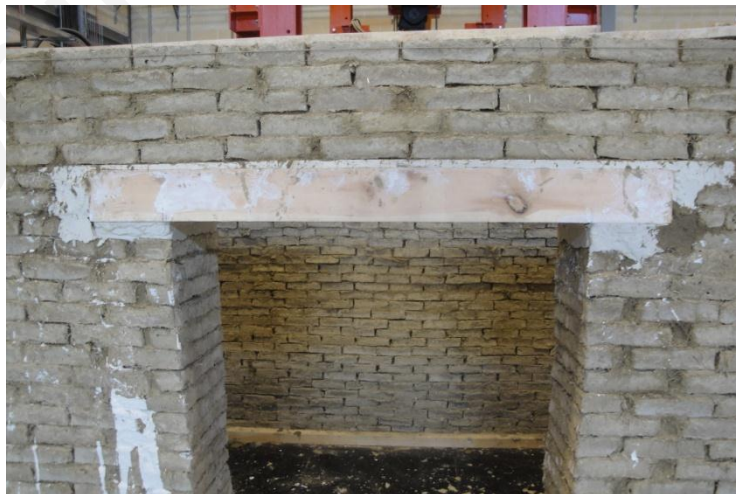
A3.8: Installation of lintels. The lintels were set into the masonry with the application of gypsum mortar. Their abutments extended approximately 150 mm into the masonry.
