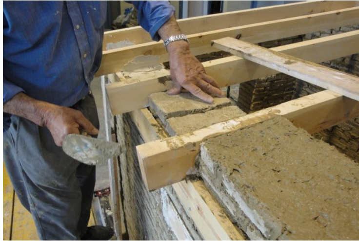
A3.9: Installation of roof rafters. Timber beams with 45 \times 90 \text{ mm}^2 cross-sections were used to span the space between the two opposite longitudinal walls. These were set into the masonry with gypsum mortar.
