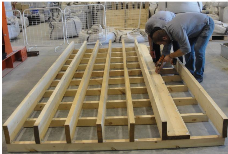
A3.1: Construction of the timber base. The cross-sections of the beams used were 50 x 100 and 50 x 200 mm 2 . The beams were orthogonally connected. Above them, wooden panels with thickness of 20 mm were fixed.
