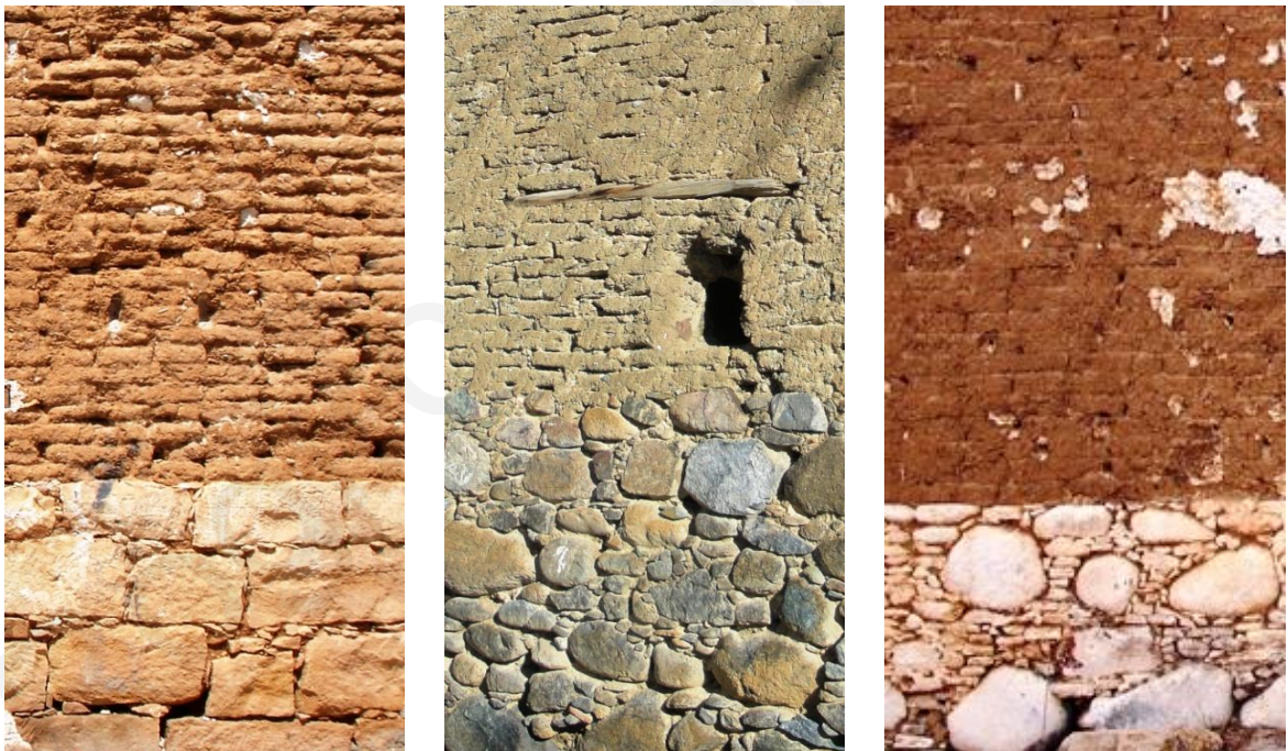
Figure 1.1: Photos of traditional Cypriot earthen dwellings showing adobe masonry walls constructed upon a rubble stone foundation. Note the variation in grain texture due to the use of different locally available materials.
