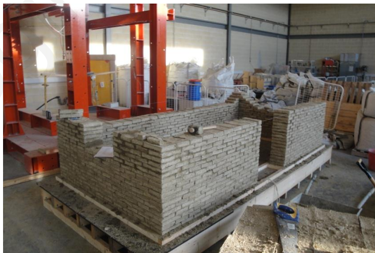
A3.5: Formation of openings. A door opening 1.10 m high and 0.70 m wide was formed on the façade and two openings 0.55 x 0.55 m 2 resembling windows were formed on the two side walls.
