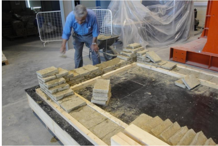
A3.3: Construction of wall corners. Connection at the cross-bricks was achieved by placing overlapping adobes.
