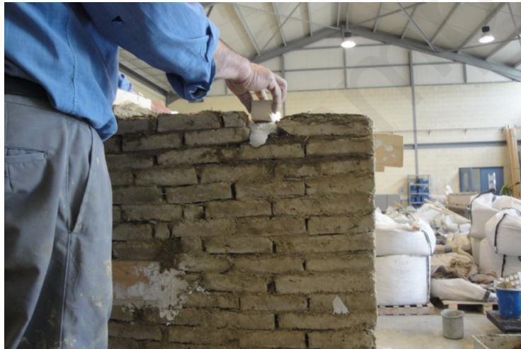
A3.10: Installation of timber wedges to prevent sliding of the inclined roof. On each side wall two timber wedges were set with gypsum mortar into the masonry. These were later nailed on the roof panel.
