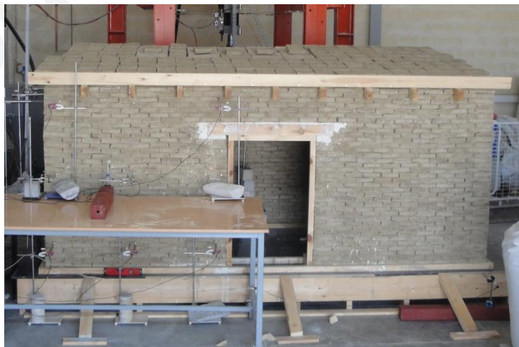
A3.11: After completing the construction of the walls, a 20 mm thick wooden panel was fixed on the roof rafters. Additional adobes were placed upon the panel to simulate the weight of roof tiles.
