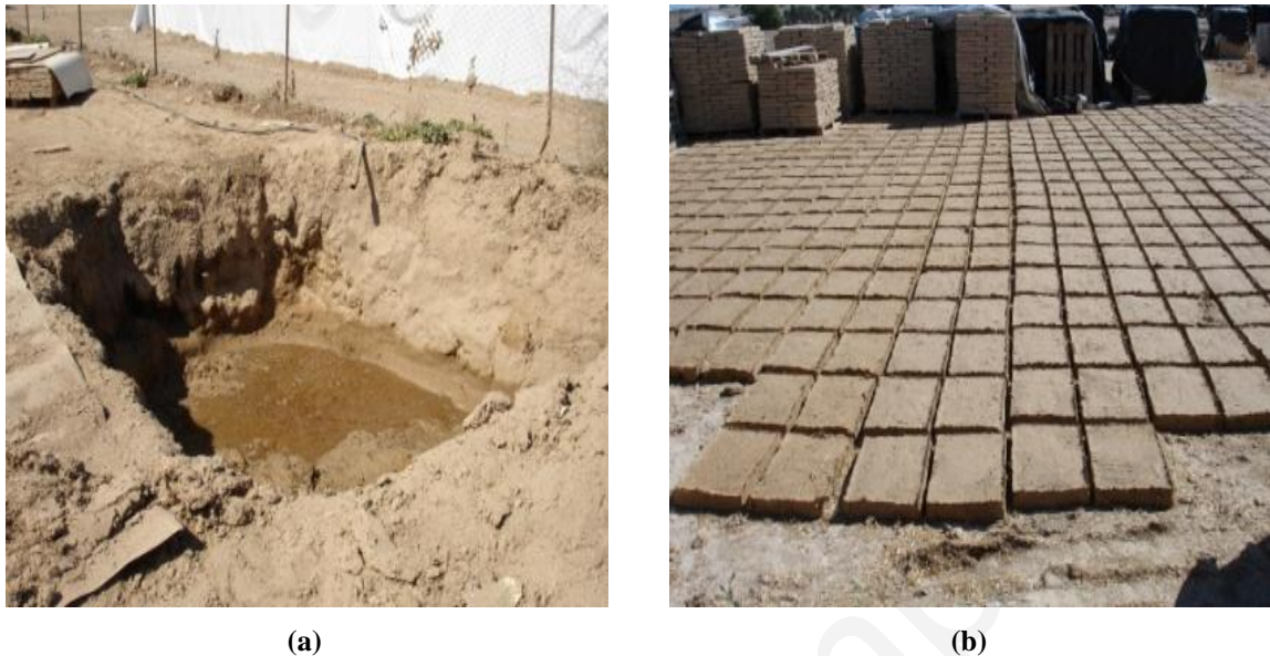
Figure 3.4: (a) Earth crater in which manufacturer Ath mixes the raw materials for the production of adobes. (b) Adobe bricks cast by manufacturer Ath laid on field ground covered with straw to dry under the sun.
