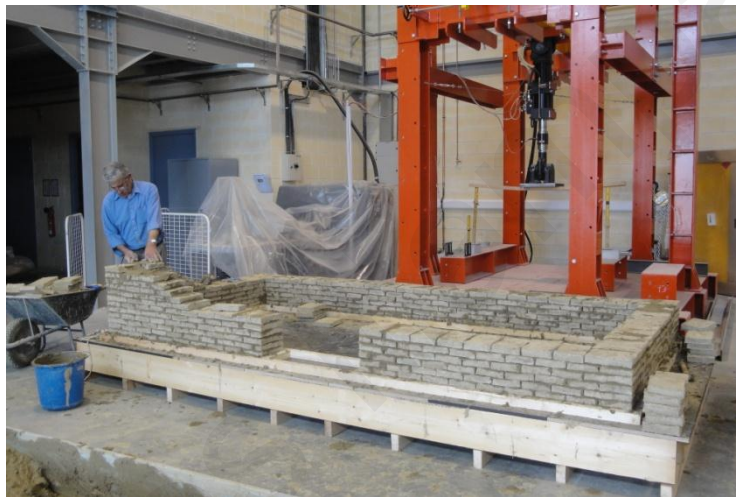
A3.4: Construction of walls. 5-6 masonry courses were first built at the corners of the structure. These acted as guides for laying the rest of adobe bricks.
