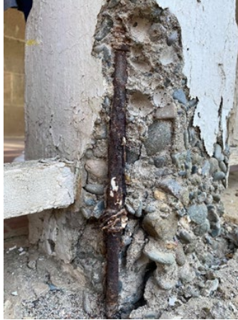
Figure 3: Cover delamination and rebar corrosion on exposed column.
