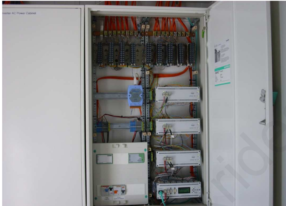
Figure 3.4. Installed data-logging and storage equipment.
