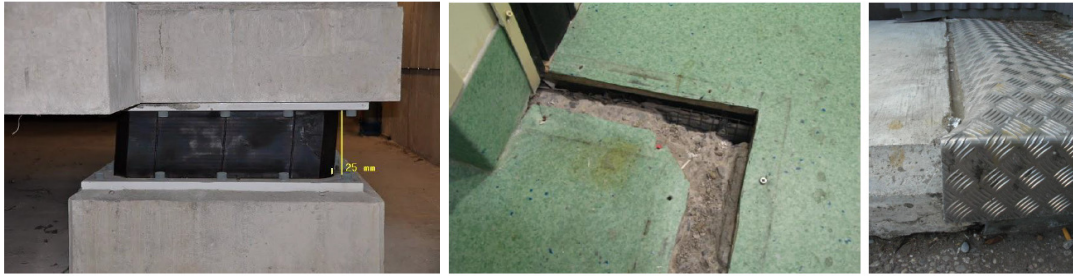
Figure 3.2 Pounding of the base-isolated Christchurch Women’s Hospital to the adjacent moat wall (Gavin and Wilkinson, 2010).
