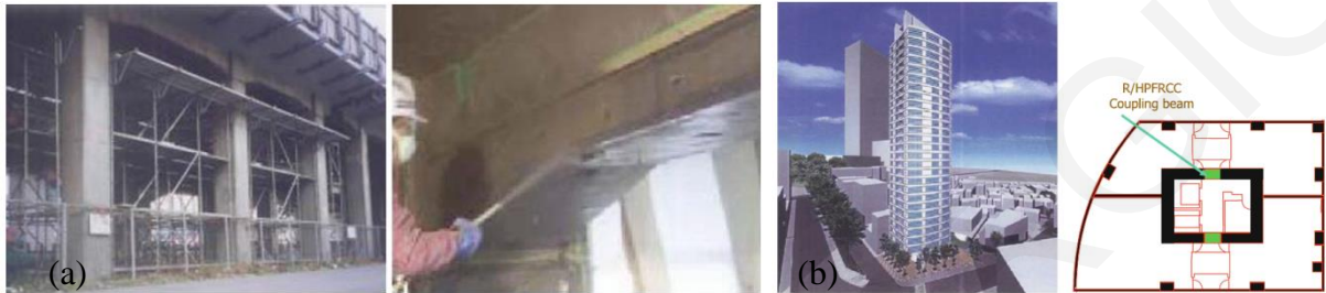
Figure 2.10 (a) Viaduct retrofitting, existing structure and direct spray construction and (b) Application of R/SHFRCC coupling beam [54]
