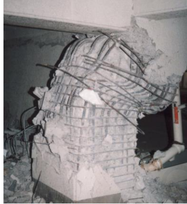
Figure 4.12: Flexural Compression Failure of a Reinforced Concrete Column
