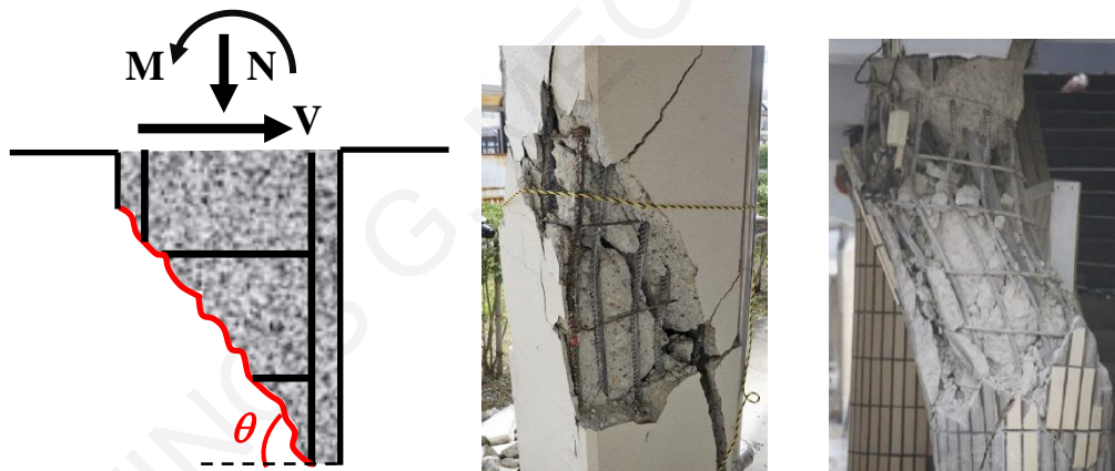
Figure 2.3: (a) Angle of inclination of the primary sliding shear crack. (b) Field evidence of shear failure
