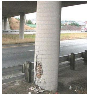
Figure 4.11: Concrete Cover Spalling of a Reinforced Concrete Column.
