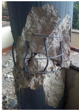
Figure 4.13: Buckling of compressive longitudinal reinforcement.
