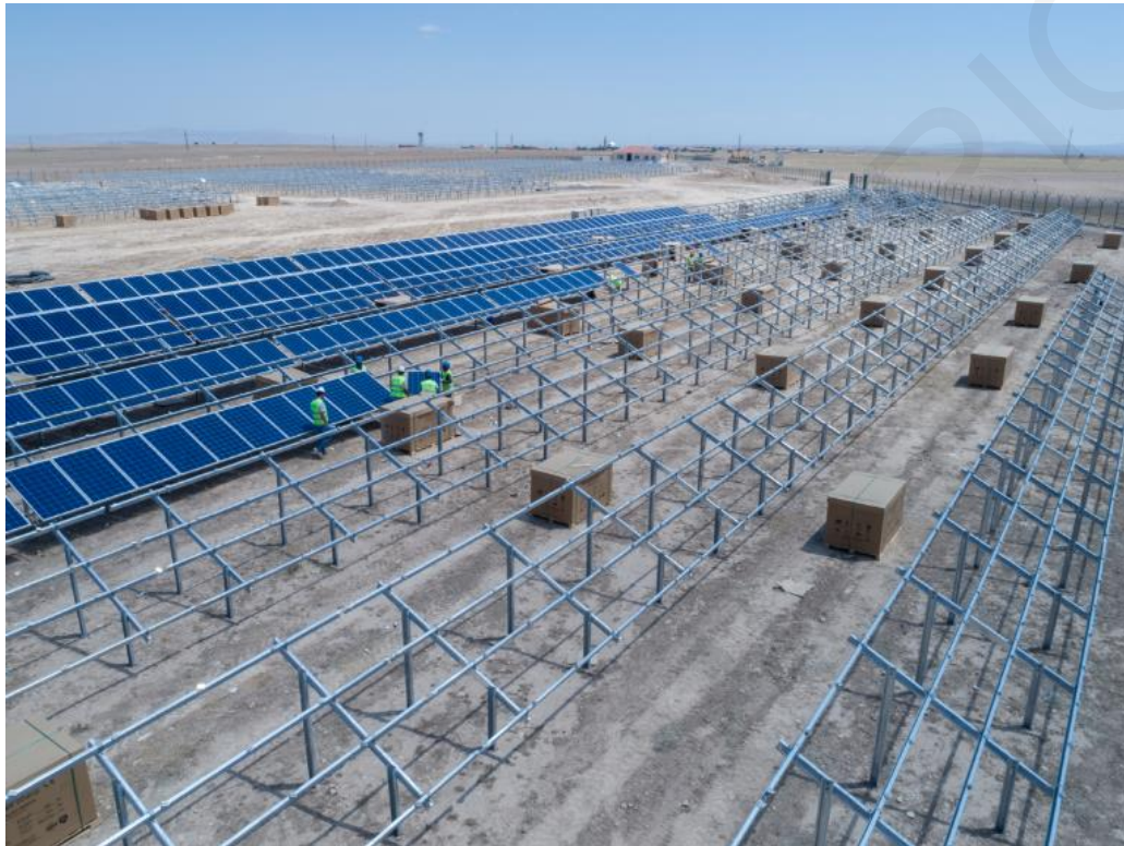
Figure 2-4: Metallic supporting infrastructure of PV modules
