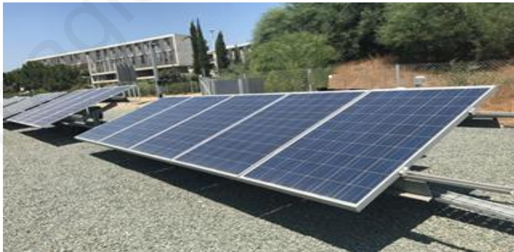
Figure 2. Poly c-Si grid-connected PV system at the OTF of the UCY.
