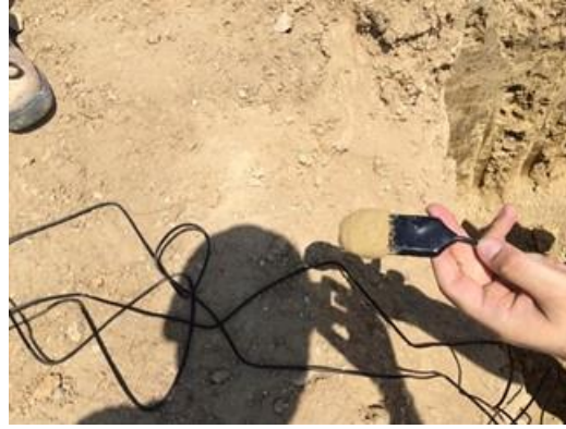
Figure 16. TEROS 21 matric suction sensors covered with remolded soil before installation.
