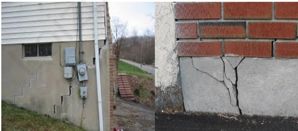
Figure 1. Examples of damage to structures due to uneven settlement of their foundations due to their construction in expansive soils.
