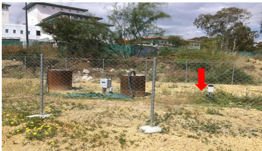
Figure 32. Completed pile heads at Site 3. Location of test pit 3 is shown with an arrow.
