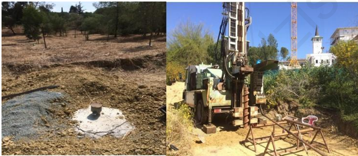
Figure 29. Open- type piezometer installed at Site 3 in borehole 3 (left) and drilling of borehole 3 (right).
