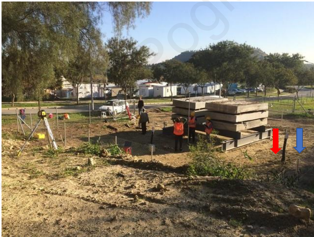
Figure 15. Site 1 with model mat foundation. Red arrow shows the location of test pit 1 and blue arrow shows the location of the wetting experiment.
