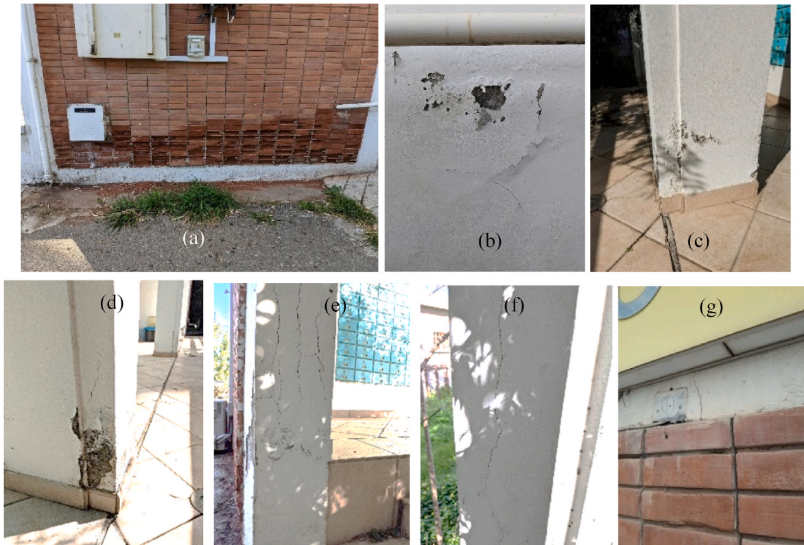
Fig. 3. Building pathology: (a) rising damp and salt crystallization damage to the fired red clay solid brick facade, (b) plaster detachment on painted infill walls, (c and d) plaster detachment on columns, (e and f) longitudinal cracks due to corrosion of the reinforcement, (g) vertical crack at the center of the entrance beam. (For interpretation of the references to colour in this figure legend, the reader is referred to the Web version of this article.)
